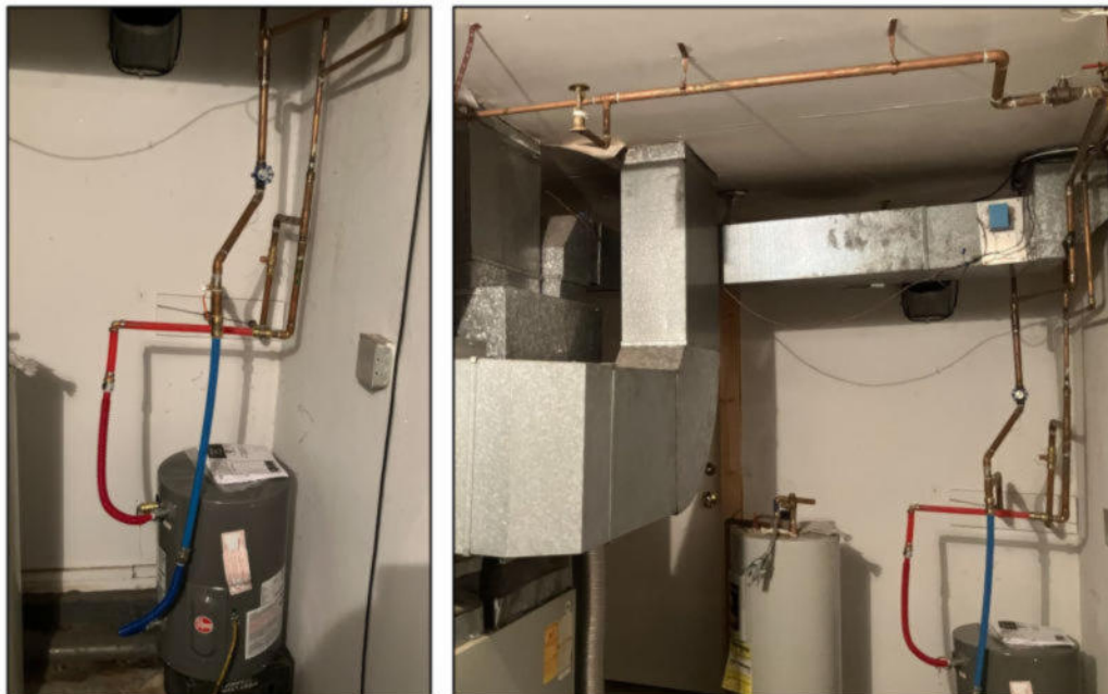
Domestic hot water heater and exposed piping
