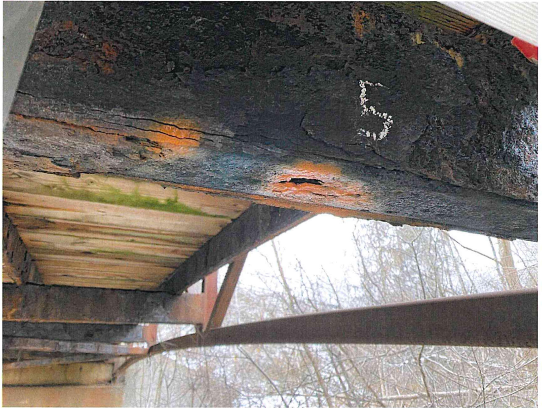
Holes in Bottom of Floor Beam 5 on Upstream end.
