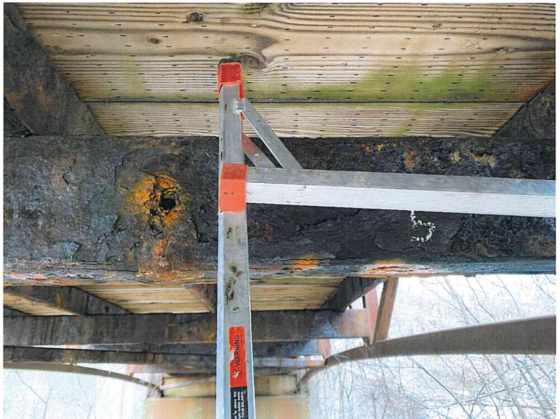
Hole in Floor Beam 5 on Abutment 2 side between stringers 1 and 2.
