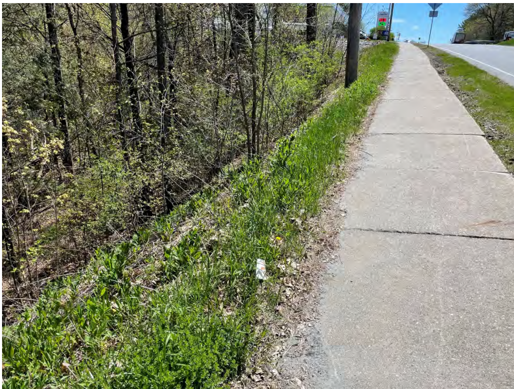
At least 10% grade on sidewalk, town lost sidewalk plow over the edge of embankment due to pitch
