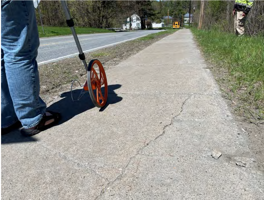
Poor uneven surface of sidewalk and it starts pitching towards the bank on right going downhill
