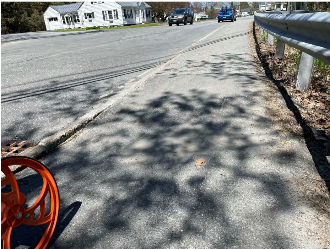
Uneven asphalt sidewalk surface creating drainage/ice ponding during rain/snow events – hazardous conditions for pedestrians.
