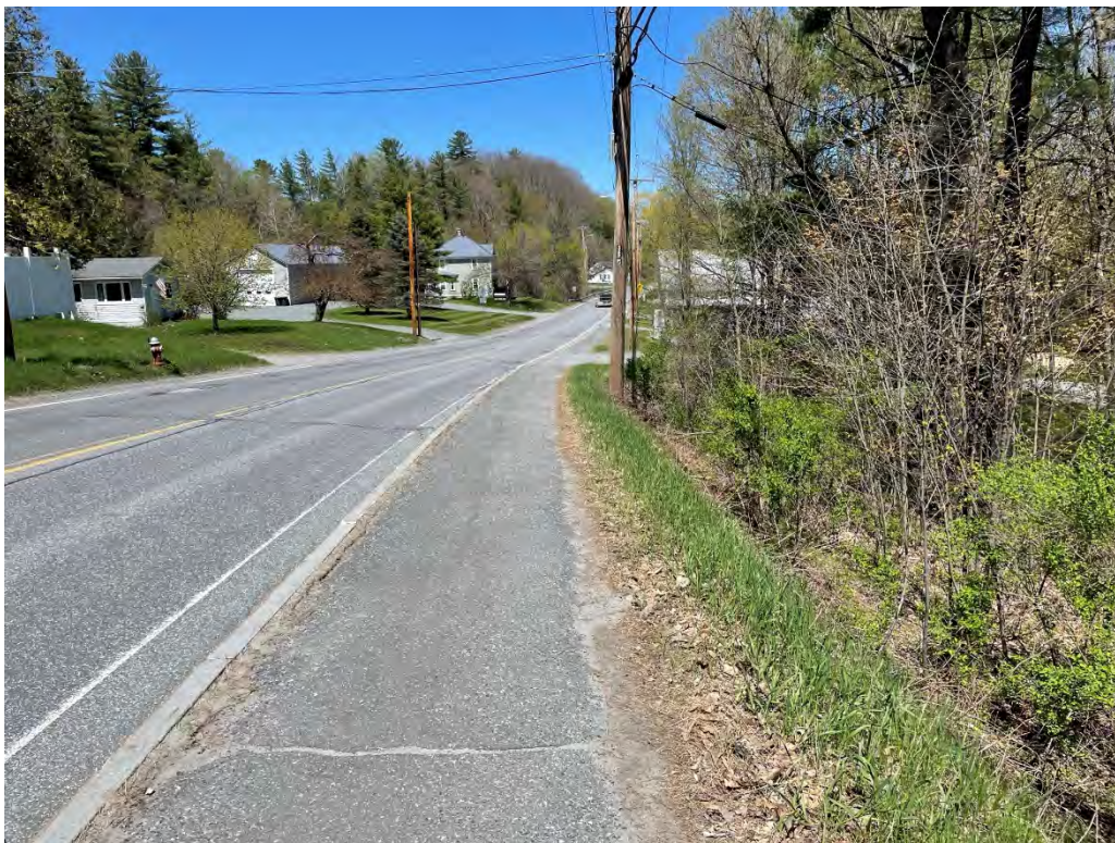
Granite curbing is nearly flush with US5
