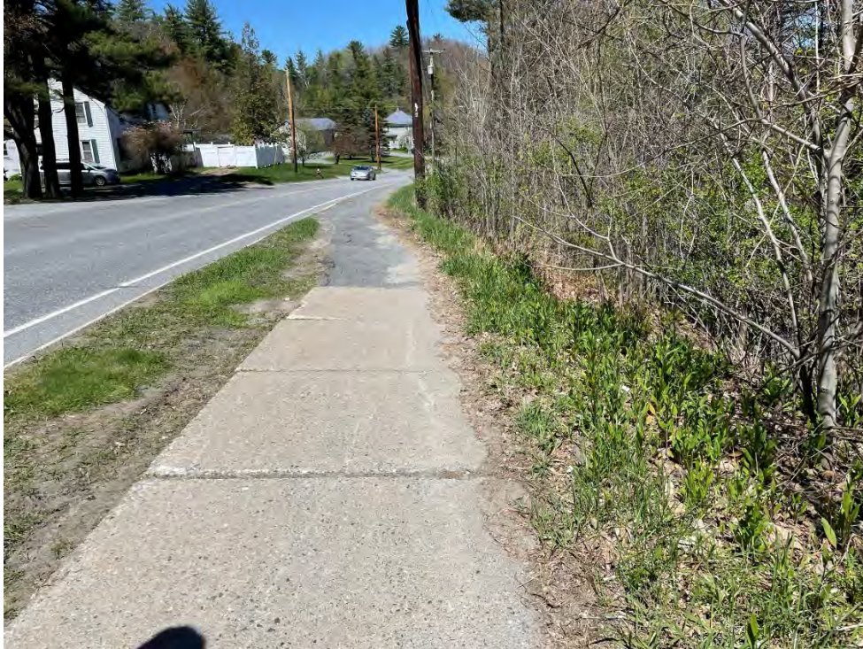
Awkward transition from concrete to asphalt sidewalk with uneven surface
